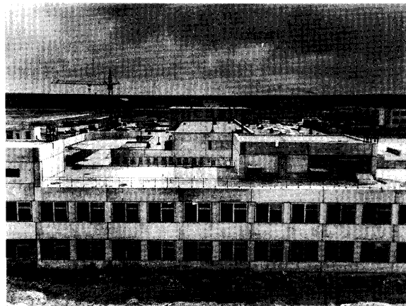
Partially constructed offices for a breeder reactor complex in the Chelyabinsk region near a Russian plutonium production facility. Construction was stopped in 1991 after a nonbinding public referendum that opposed the building of new reactors.
